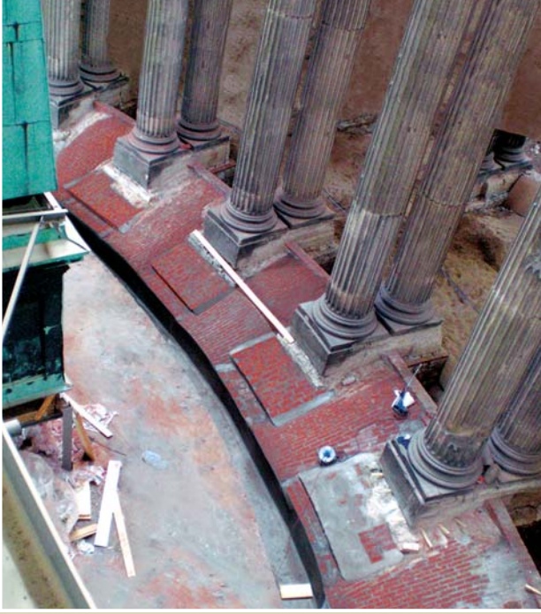
Colonnades of the new palace at Schloss Sanssouci in Potsdam – restored by Spesa
