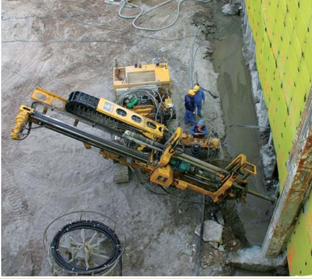
Anchor works as part of the reconstruction of the Wusterwitz canal lock
