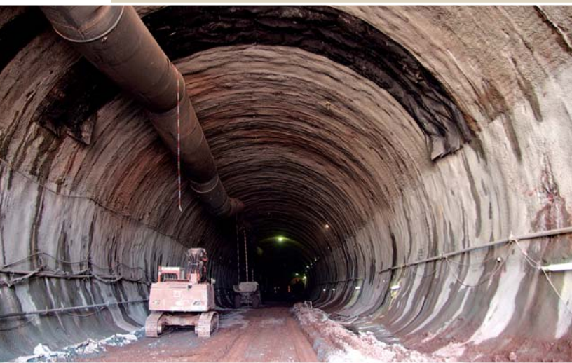
Müss tunnel on the new Nuremberg-Erfurt rail link – constructed by Schachtbau Nordhausen
