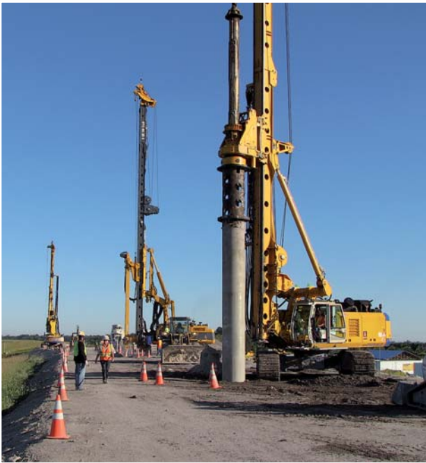
CSM cut-off walls to remediate the Herbert Hoover Dike around Lake Okeechobee in Florida
