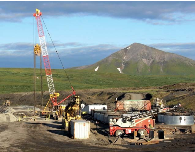
Cut-off wall for the Red Dog Mine in Alaska
