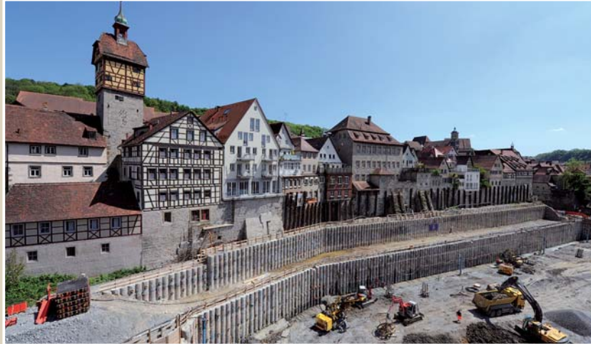
Piled walls as retaining structure at the Kocher Quarter in Schwäbisch Hall
